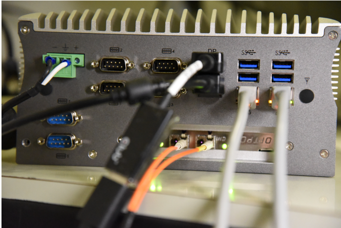
Figure 8: Rear side cabling of the PicoSys 2614 computer. The left of the two grey RJ45 Ethernet cables is connected to the wall (MPIA Internet), the right is connected to the switch. One of the two orange fibers from the ROE is plugged into CHAN1, the other into CHAN0 of the OPTPCI. The sending connectors of CHAN0 and CHAN1 are not used. To get nonzero data, the fiber head with the yellow cap is to be inserted into CH1, the fiber with the white cap into CH0 (with the setup on the ROE in 2021-02).
